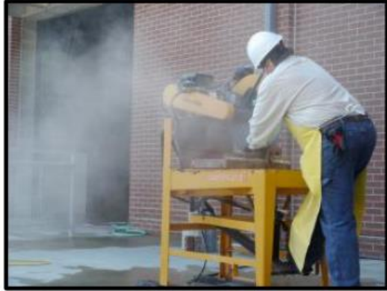
✘ No Engineering Controls
