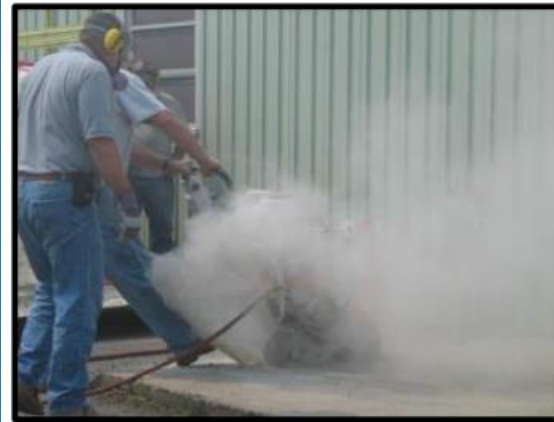
✘ No Engineering Controls
