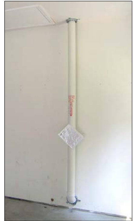
An example of a radon-control vent pipe.
