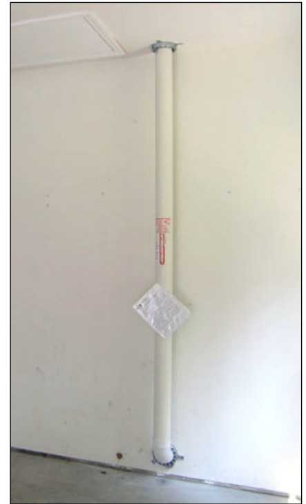
An example of a radon-control vent pipe.
